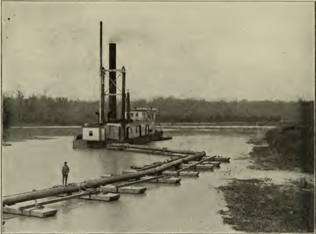
FIG. 34. 20-INCH HYDRAULIC DREDGE, VICKSBURG, MISS., MAKING NEW CUT TO RESTORE RIVER NAVIGATION TO THE CITY.
